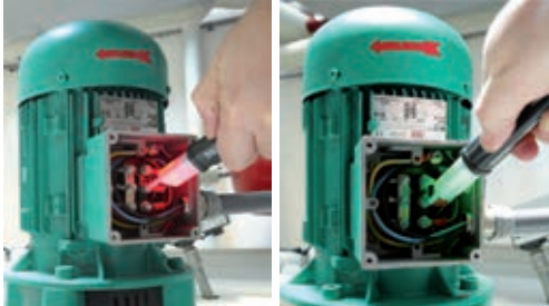
Incorrect phase sequence
