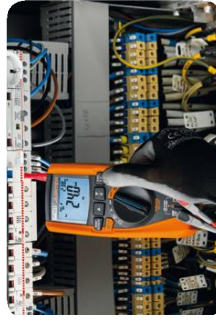
RCD tripping time and current measurement.
